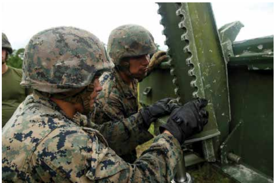
ESB Mairnes assembling a medium girder bridge. (Photo by LCpl Tyler Stewart.)
