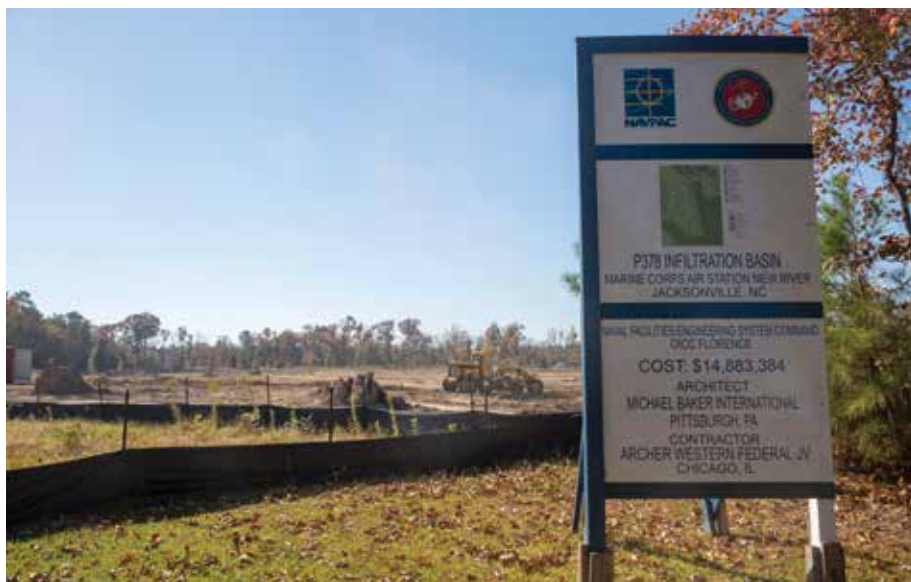
This water infiltration basin will provide MCAS New River with 190 acres of impervious area and will be able to handle the first two inches of storm water runoff. This decreases the need for stormwater ponds on the flightline, reducing Bird/Aircraft Strike Hazard (BASH) concerns by eliminating the bird habitat. (Photo by Cpl Christian Ayers.)
