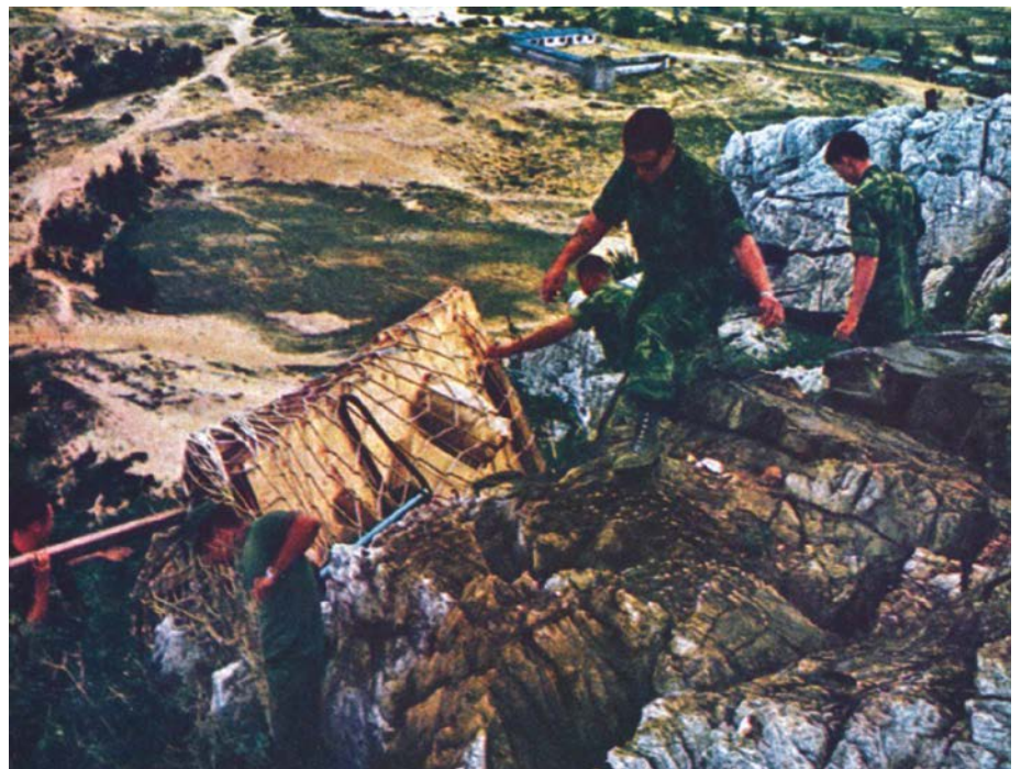
Marines from the 1st Engineer Bn erected sturdy hootches on the mountain's wind-swept summit.
