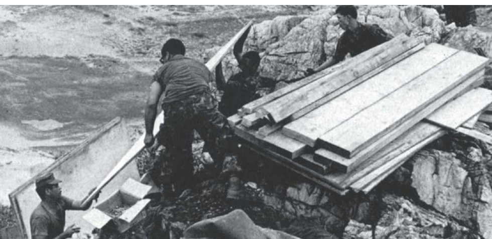
A crew of Marine engineers was quickly initiated to the dangers of living on the Crow's Nest when a pallet of lumber was deposited precariously on the side of the 400-foot mountain.
