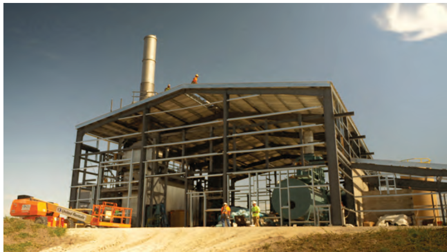
The new cogeneration (CHP) plant at MCRD Parris Island under construction in July 2018. (Photo by author.)
