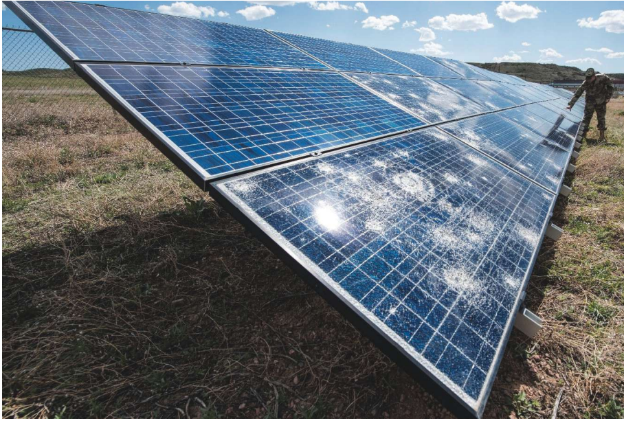
2019-NREL researcher Kate Anderson and the Fort Carson garrison commander, COL Wortlinger, review a photovoltaic array damaged by hail. Fort Carson was hit with a record hail storm, resulting in damage to 25–50 percent of the photovoltaic systems on site. Through funding from the U.S. Department of Energy’s Federal Energy Management Program, NREL evaluated long-term safety and performance issues, developed lessons learned on how to address damage, and developed guidelines on how to evaluate contractor solutions. (Photo by Dennis Schroeder/NREL—www.)
