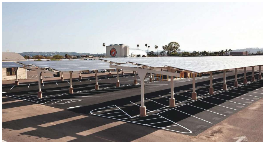
Since 2008, NREL has partnered with MCAS Miramar, helping it become more renewable energy resilient. MCAS Miramar developed a microgrid powered by solar, landfill gas, natural gas, and diesel fuel, as a redundant power option supporting critical services. (Photo by NREL at www.mil.gov .)
