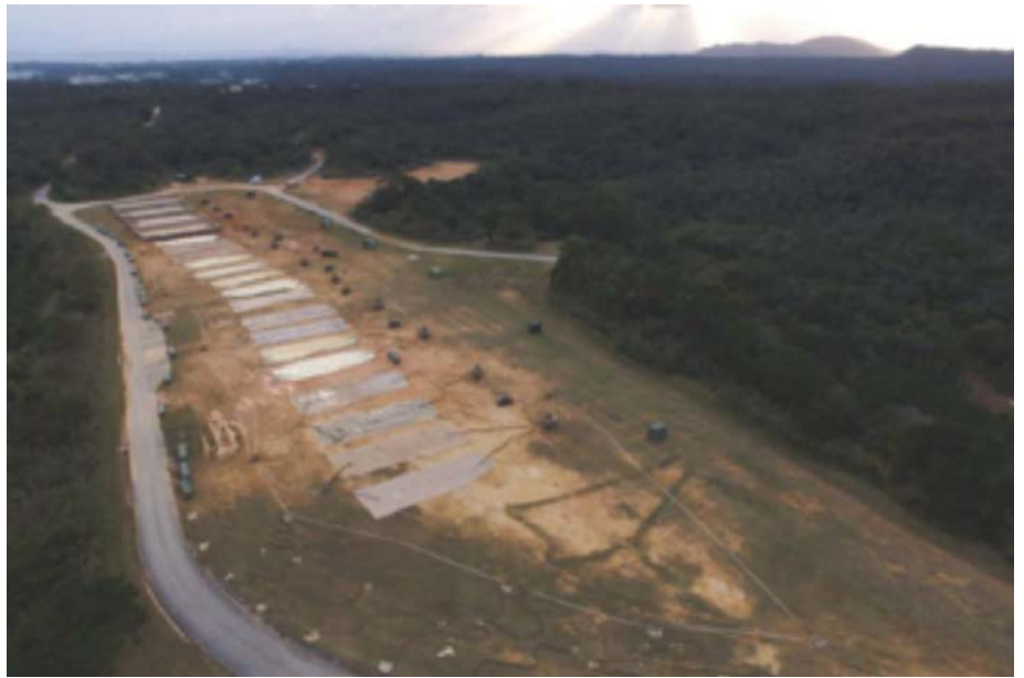
One million-gallon fuel farm, 9th Engineer Support Battalion, Bulk Fuel Co, Central Training Area, Okinawa, Japan (January 2017). (Photo by LCpl Roland James.)
