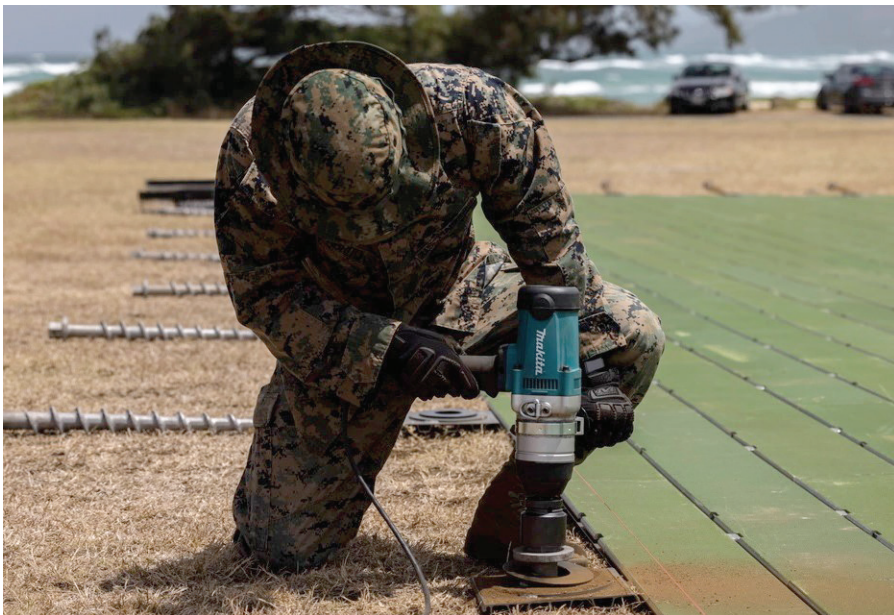
A Marine Corps expeditionary airfield technician with MWSS-174 installs PE-36 anchors for prefabricated surface aluminum flat top nested airfield matting while training for expeditionary advanced base operations. (Photo by LCpl Hunter J. Jones.)
