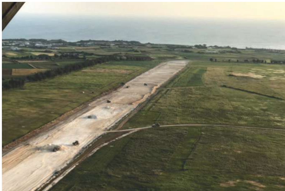
LEEG engineers will be critical to theater development creating expeditionary advanced bases, advanced naval bases, and expeditionary airfields (depicted above on Ie Shima Island, Okinawa Prefecture). (Photo credit: 9th ESB, III MEF.)
